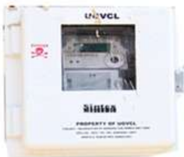
Smart Meter installed at consumer end in entire Modhera
