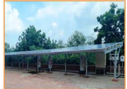
50kV Solar Parking Structure near Modhera
